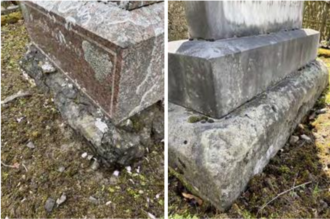
Figure 10 - Memorial adhesive failed between each component
