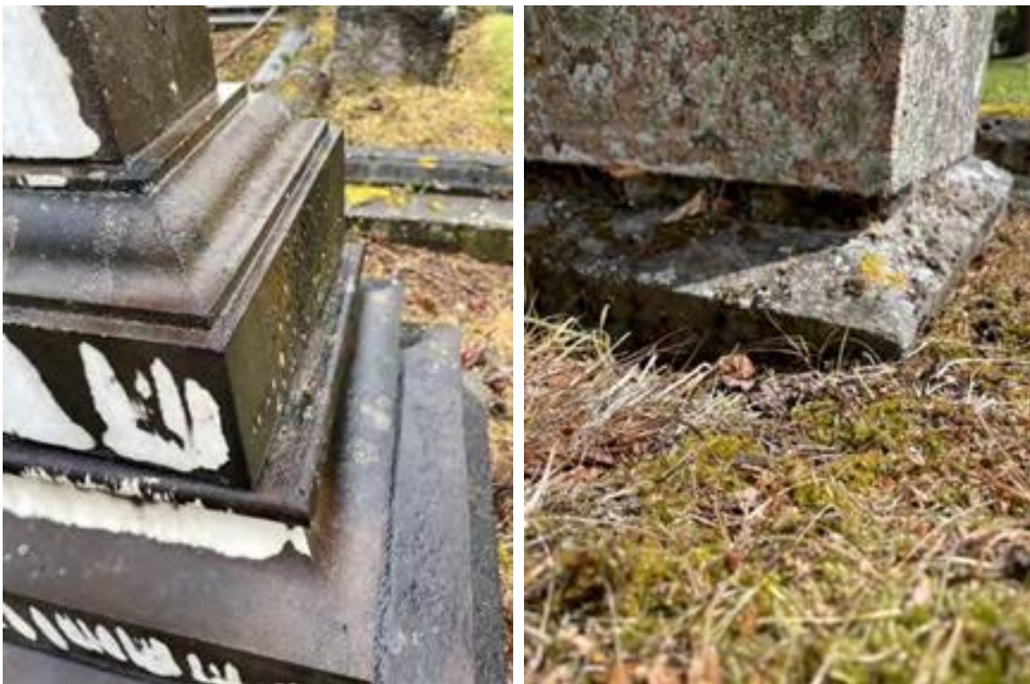
Figure 9 - Memorial joints loose/wobble and memorials have shifted on their base due to adhesive failure and lack of internal supporting rods
