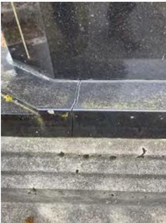
Figure 7 - Adhesive on joints failed and cracked base, memorial loose
