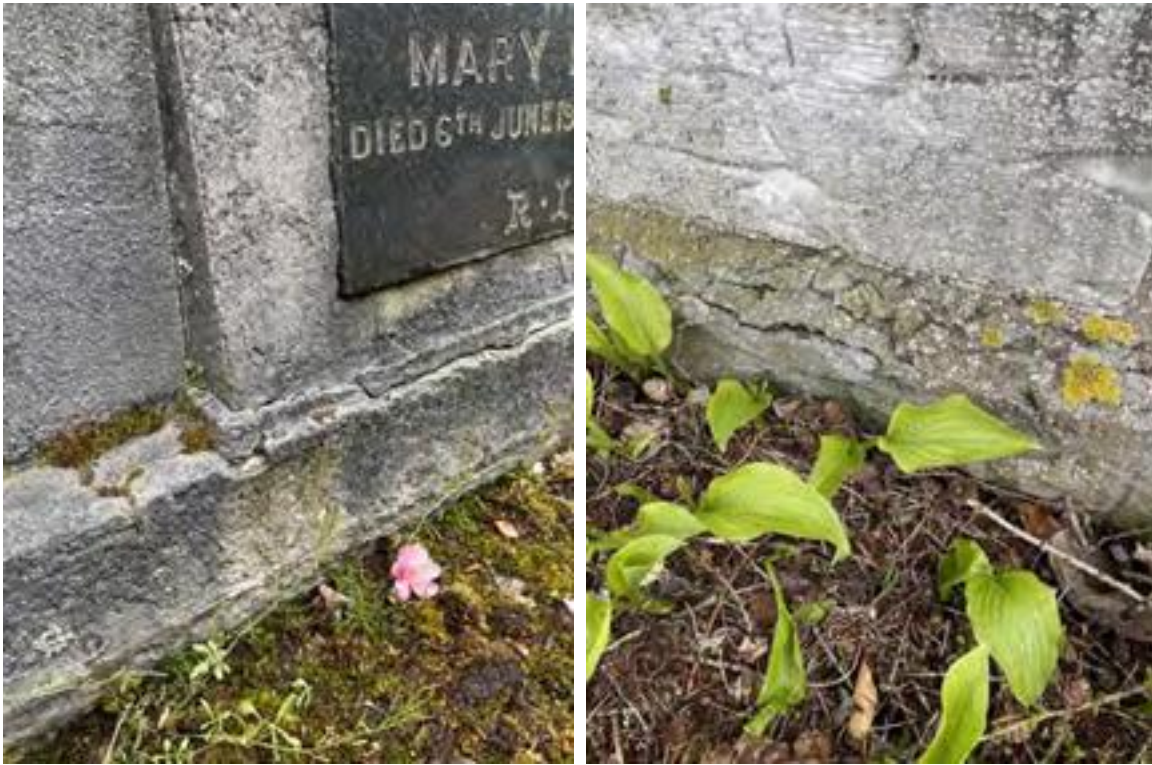
Figure 8 - Loose joint material causing memorial to wobble on base
