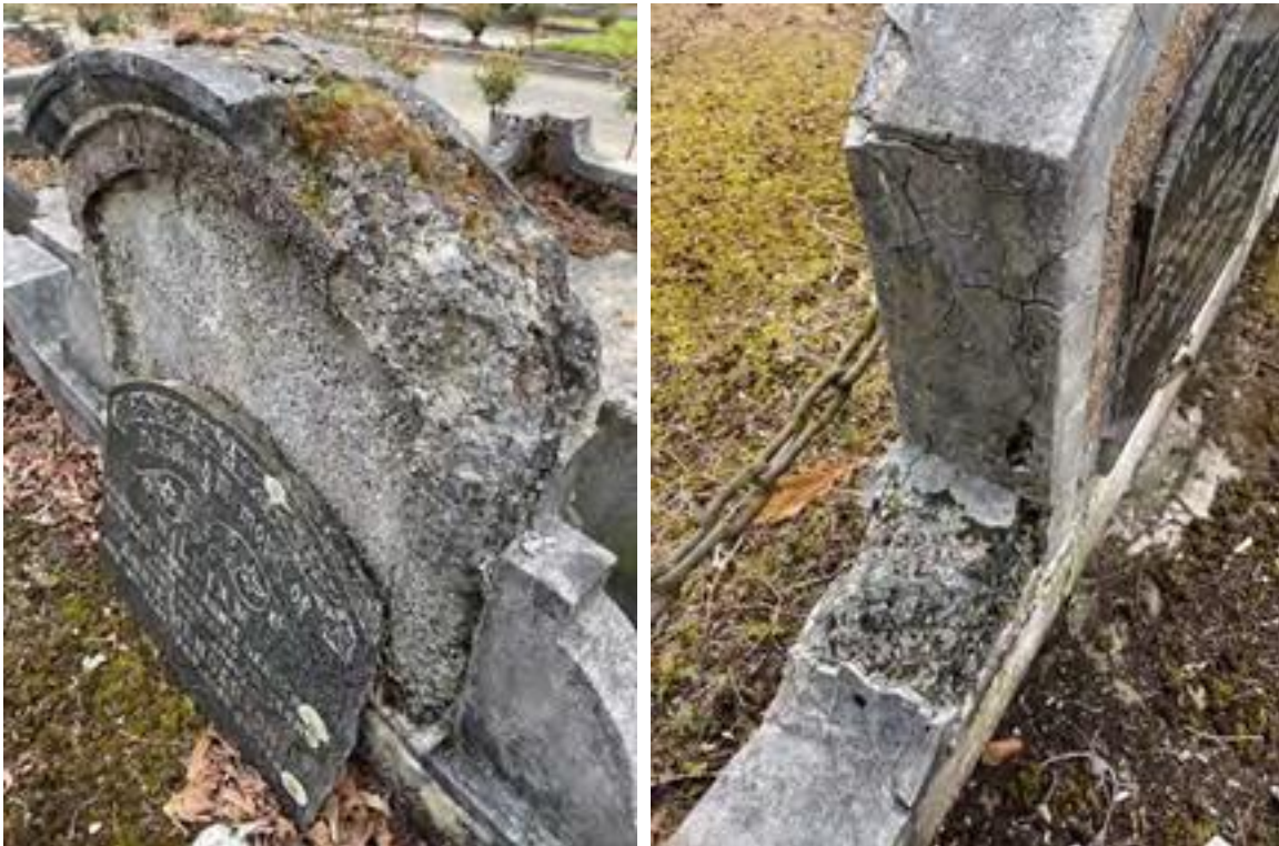
Figure 1 - Plaster covered memorial showing signs of failure and weak joints that move. Upright memorial components loose.
