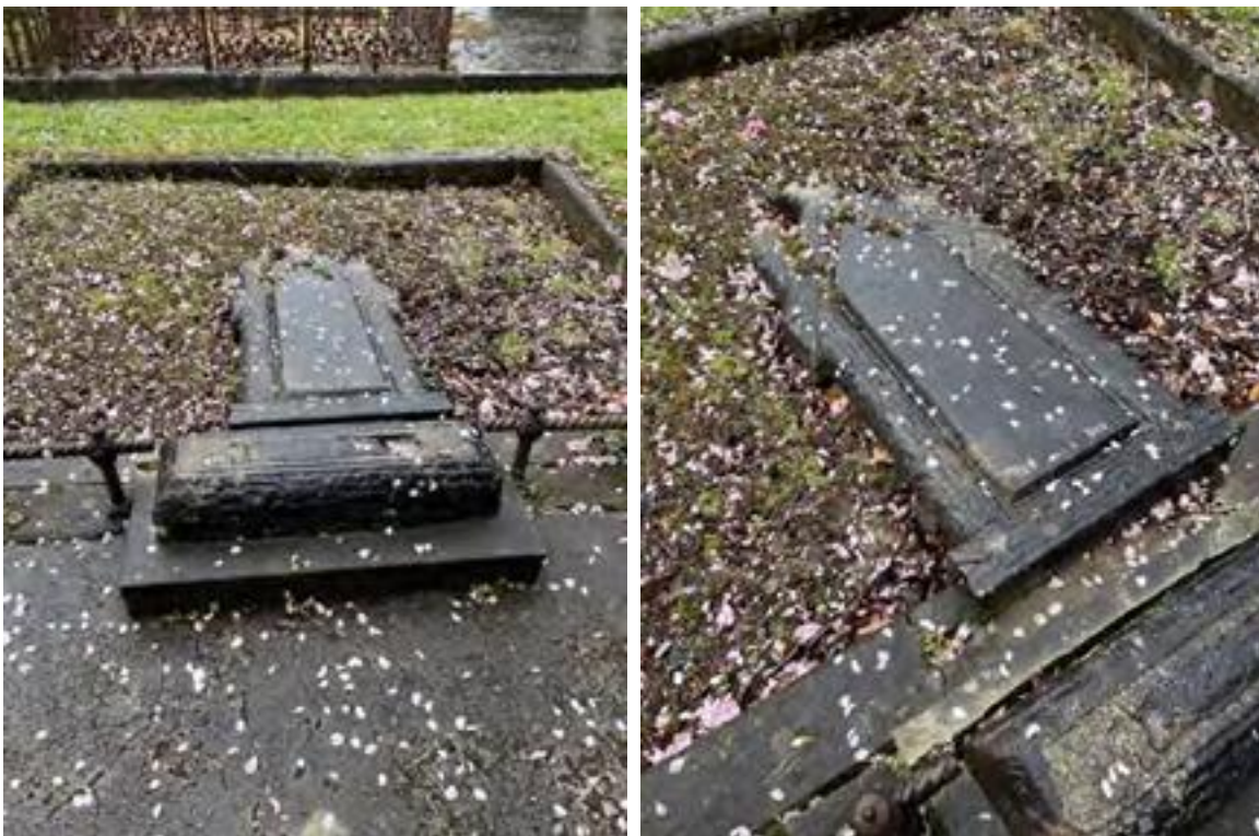
Figure 11 - Joint failure causing memorial to fall.
