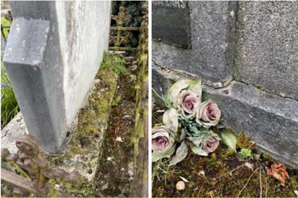
Figure 6 - adhesive on joints has failed causing a loose memorial
